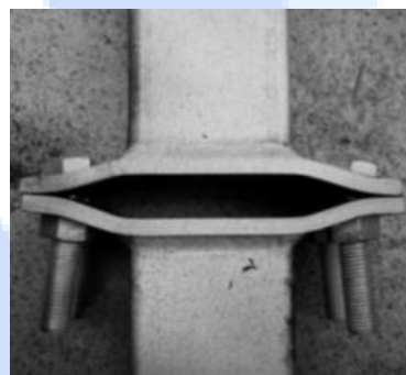
Figure 3. Bolt yielding and plate separation failure (Lacey et al. 2019)
