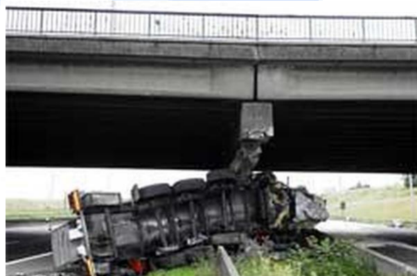
Figure 2. Damaged pier after truck collision
